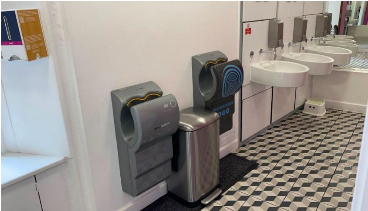
Floor 1: Hand dryers in toilets (will be turned off)
